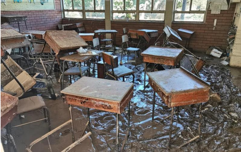
A mud-filled classroom in eThekweni, KwaZulu-Natal caused by unprecedented high rainfall and flooding on 11 April. ©Government of South Africa/2022
